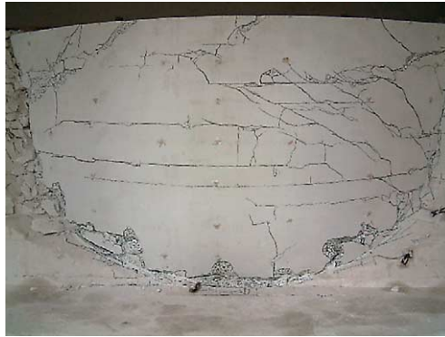
Fig. 14. Failure of upstream of Xiluodu arch dam with seven times upstream water pressure overloading (physical modeling test).
